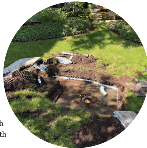
A roof champion investigated a leak at this exposed roof drain on an inverted roof membrane assembly with landscape overburden
