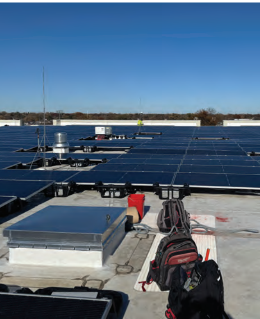
This solar array is an example of when a roof champion can review construction detailing.
