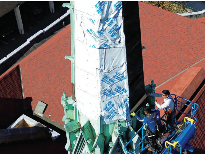
After the copper was removed, the steeple was temporarily wrapped in underlayment.
