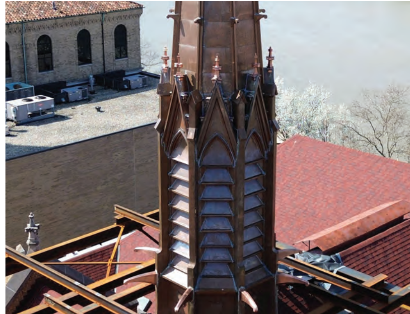
Special attention was given to seam alignment, solder joints and ornamental profiles to ensure a historically accurate restoration.
