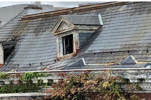
Before renovations, the building was in an advanced state of deterioration.
