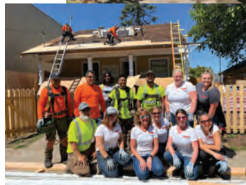
Bliss Roofing partnered with Home Builders Foundation and National Women in Roofing Oregon Council to provide a new roof for Project Homeless Connect.
