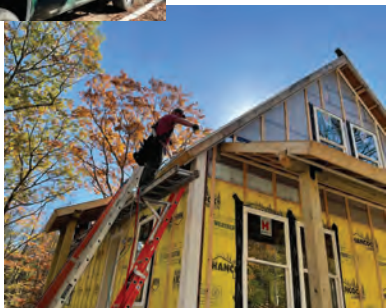
Industrial Roofing partnered with Beacon Building Products to install a new roof system on a house for Habitat for Humanity.
