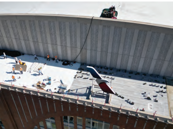
Top to bottom: Safety training sessions were held with Dallas police, arena personnel and KPost Company team members to coordinate helicopter operations; the helicopter made 140 trips to lift the bulk of materials to the roof; roof system installation in progress
