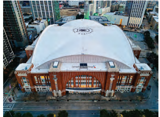
Top to bottom: KPost Company team members apply the liquid roof membrane; aerial view of American Airlines Center’s newly completed roof systems
