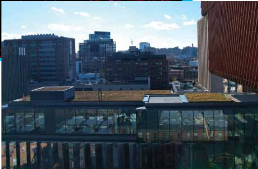
The Greenwood Industries crew installed 32,000 square feet of vegetative roofs on multiple levels.
