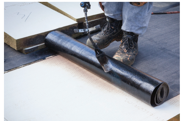
Photo: Installing stone wool insulation between the deck and cover board under the roof membrane or deck can help with sound absorption.
