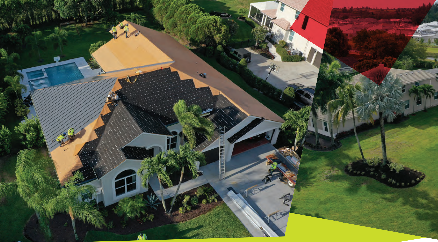
Left and middle: The Moss family's roof system changes from concrete tile to metal components.
