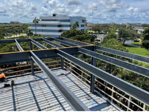
Part of the theater's new structure was built over the existing structure.
