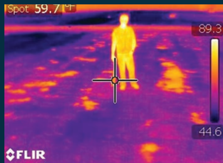
An infrared image of a thermal anomaly marked on a rooftop (a person is in the image for scale)
