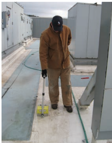
A nuclear gauge in use on a rooftop. Photo courtesy of White Glove Building Maintenance, Salem, Ore.
