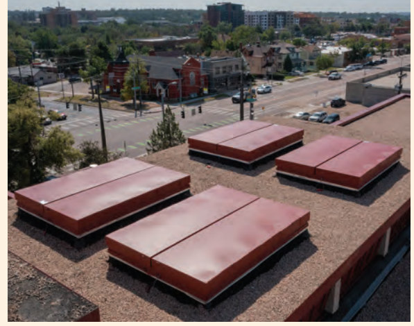
The newly installed acoustical smoke vents
