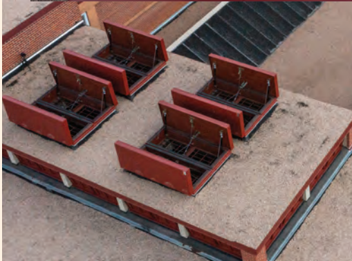
Portions of the existing concrete roof deck were removed to provide openings for new smoke vents.
