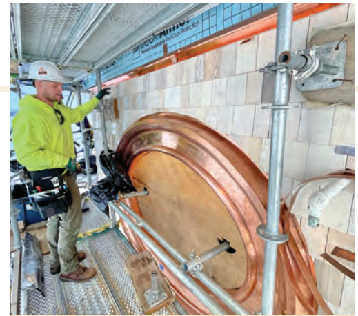
Custom-manufactured copper window architraves were fitted and installed around circular window openings.
