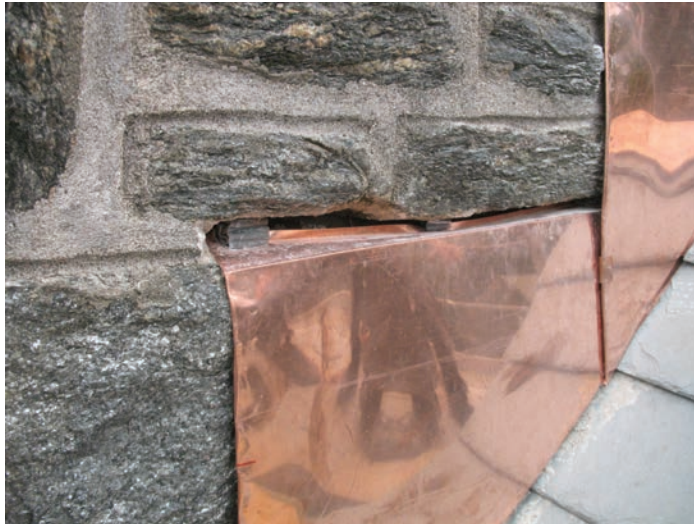
Photo 2: This reglet will have to be redone. The reglet flange of the counterflashing is too narrow given the depth of the reglet cut in the mortar joint. The kink below the lead wedge on the right indicates the reglet slopes into the wall in this area. The lead wedges also are set too close to the surface of the joint, allowing for insufficient coverage of the yet-to-be-installed mortar fill.
