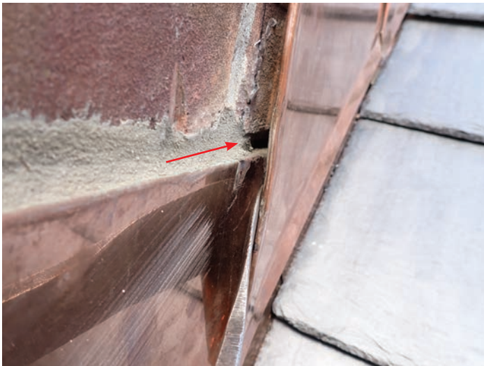
Photo 3: Lack of coordination between the roofing contractor and masonry contractor led to the concealed portion of the underlying counterflashing's reglet not being filled with mortar before installation of the overlying counterflashing (red arrow).
