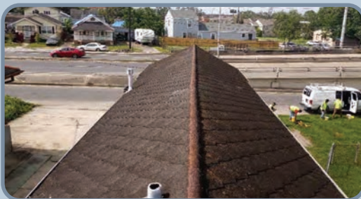
Damaged roof before Stormseal
