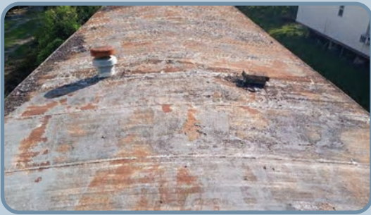
A hurricane-damaged roof before Stormseal
