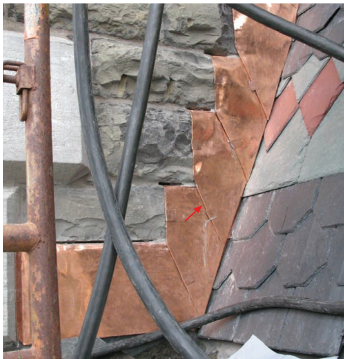
Photo 1: The lower corners of these soft copper counterflashings have been angled back toward the roof to help minimize their apparent size (red arrow), and their bottom ends are hemmed and loose-locked together to help prevent outward displacement.
