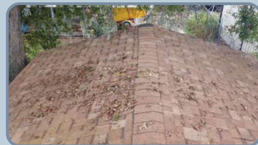
Damaged roof before Stormseal
