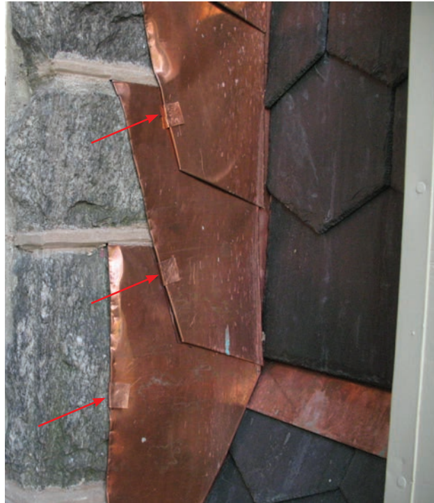
Photo 4: Close-up of 20-ounce copper clips used to help secure counterflashings
