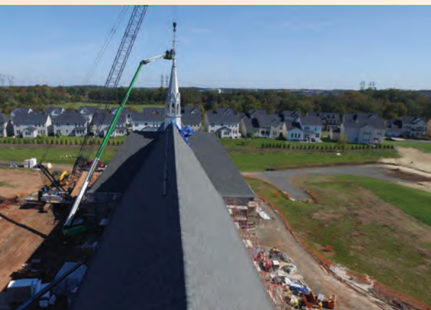
Top to bottom: The roof was designed with a sweep across the bottom where the slope transitions from 18:12 to 2:12 along a curve; the church during construction; after the steeple was tied in, a stainless-steel cross was added.
