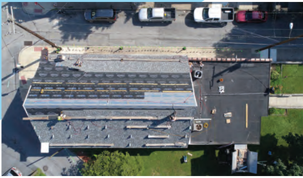
GSM Roofing, Ephrata, Pa., gifted a new roof system to Bethel AME Church, Lancaster, Pa., through its annual Great Roof Giveaway.
