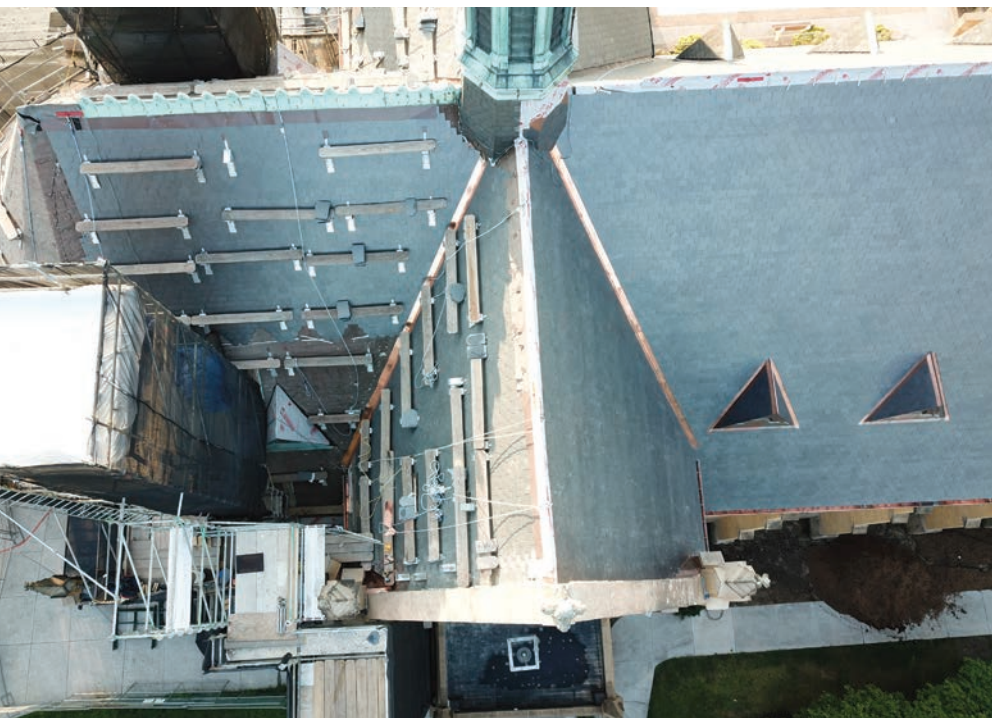
The project's second phase of work included installing a new slate roof system with ornamental copper. Each piece of slate was hand-cut to match its original size and shape.
