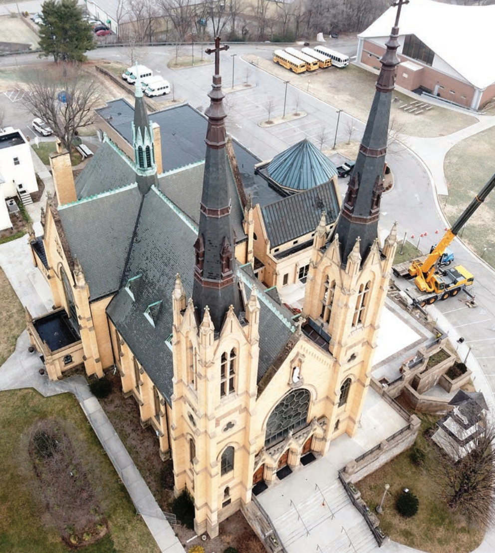
Workers removed and replaced the steeples simultaneously following the original 1902 architectural design but used steel instead of wood for the framing.
