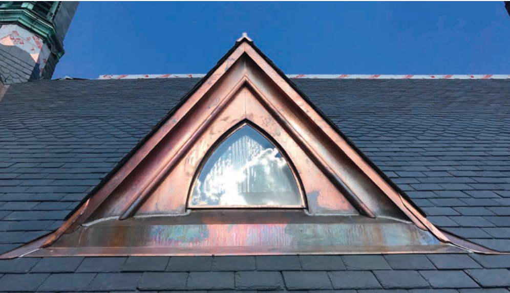
The Durable Slate Company craftsmen hand-soldered each piece of copper to ensure a watertight fit.
